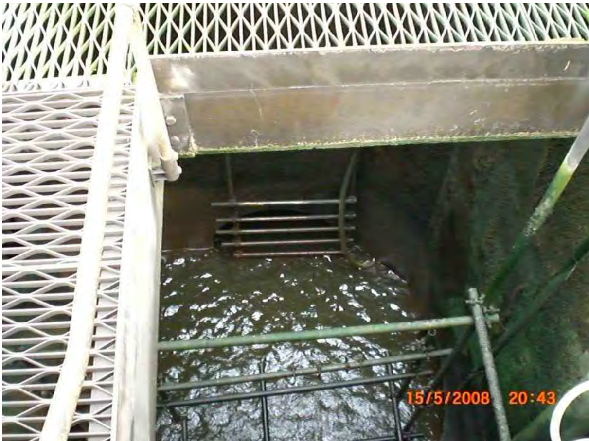
Above. Exposed collection chamber and start of the underground concrete pipeline at the penstock weir area
