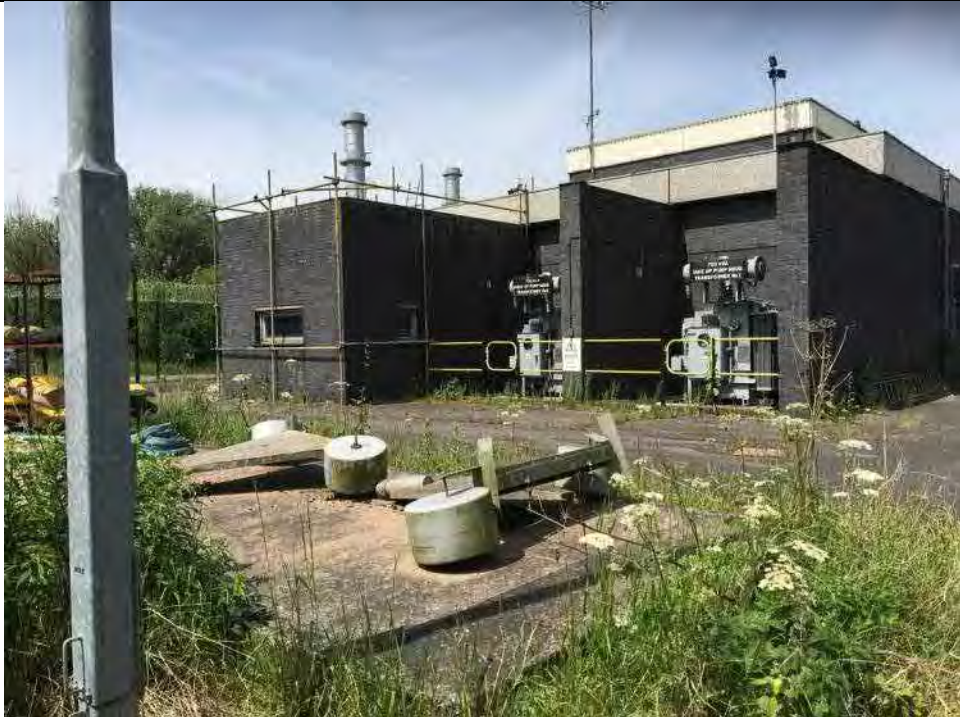
Photograph 27 | Main power station abstraction pumphouse
